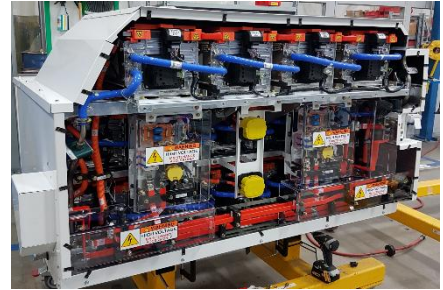
Figure 54 Low Voltage Distribution Box
