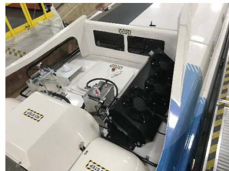
Figure 33 BEB expansion tanks
